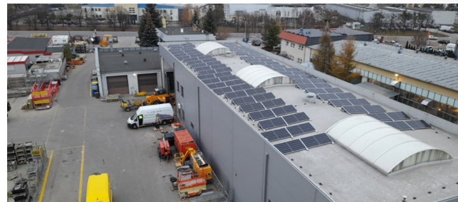
Solar farm - Poland
