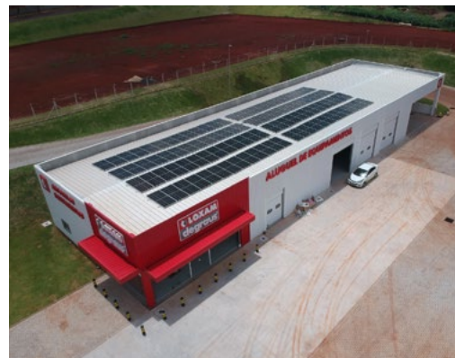
Solar farm - Araquara branch, Brazil
