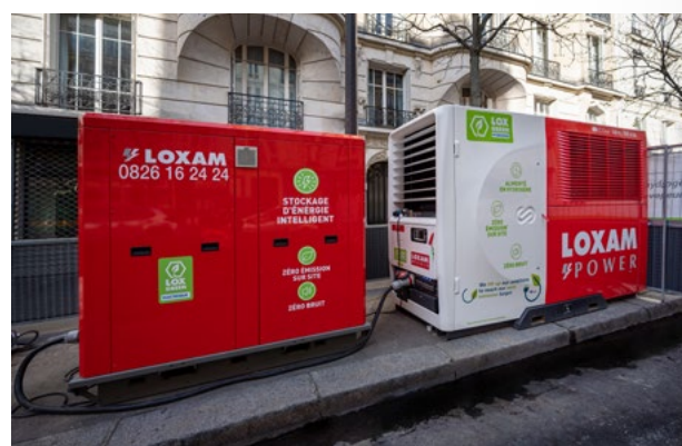
90kWh power bank and hydrogen power generator
